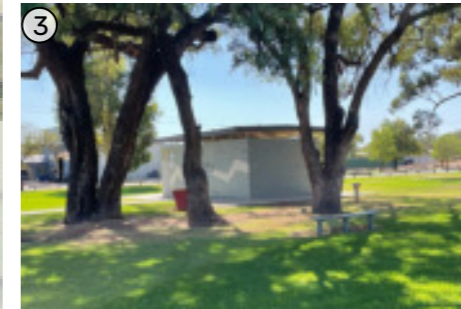
Existing toilets - Lack of accessible facilities - Dated appearance
