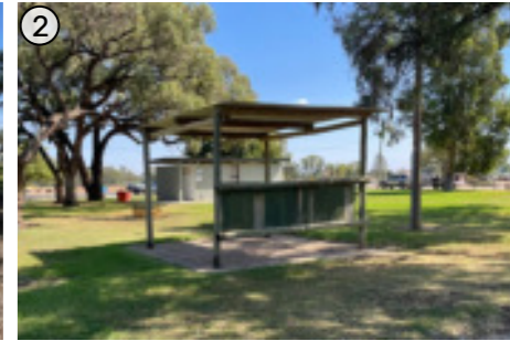
Existing Shelter - Dated, need to be replaced
