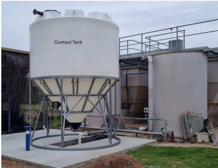
Contact tank & plinth July 2025
