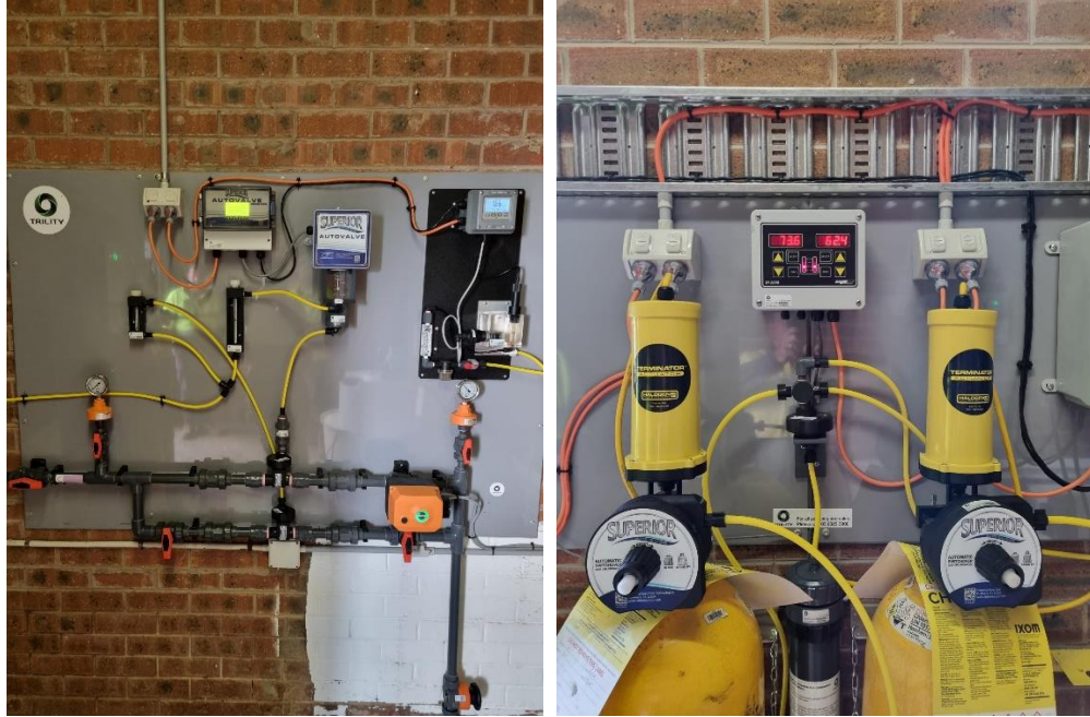
September 2025 new chlorine gas monitoring equipment
